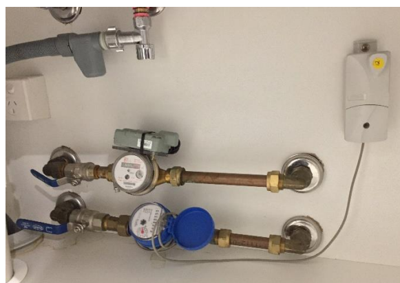
Cold and hot water sub-meters with remote reading devices. Hot water meter in this case is read by the Corporation's gas provider (for gas billing purposes), the cold water meter is read by SWS. We obtain hot water reads from the gas provider to bill owners for total water usage
